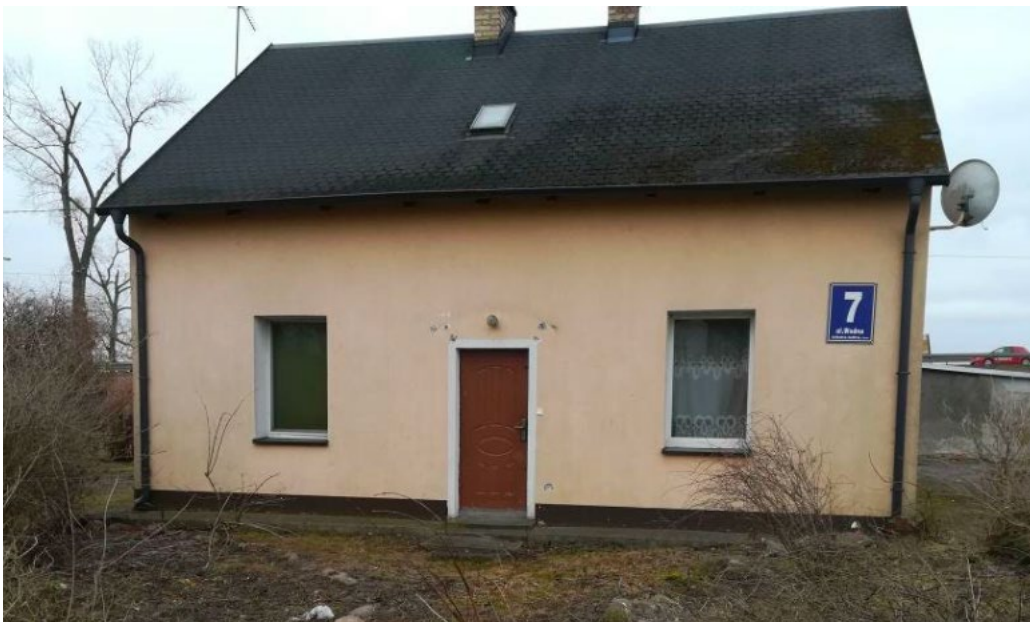
Figure 46. The building at 7 Wodna Street, Nakło nad Notecią / Source: Local Revitalization Program for the Town and district of Nakło nad Notecią for the years 2016 - 2023, p. 31.
